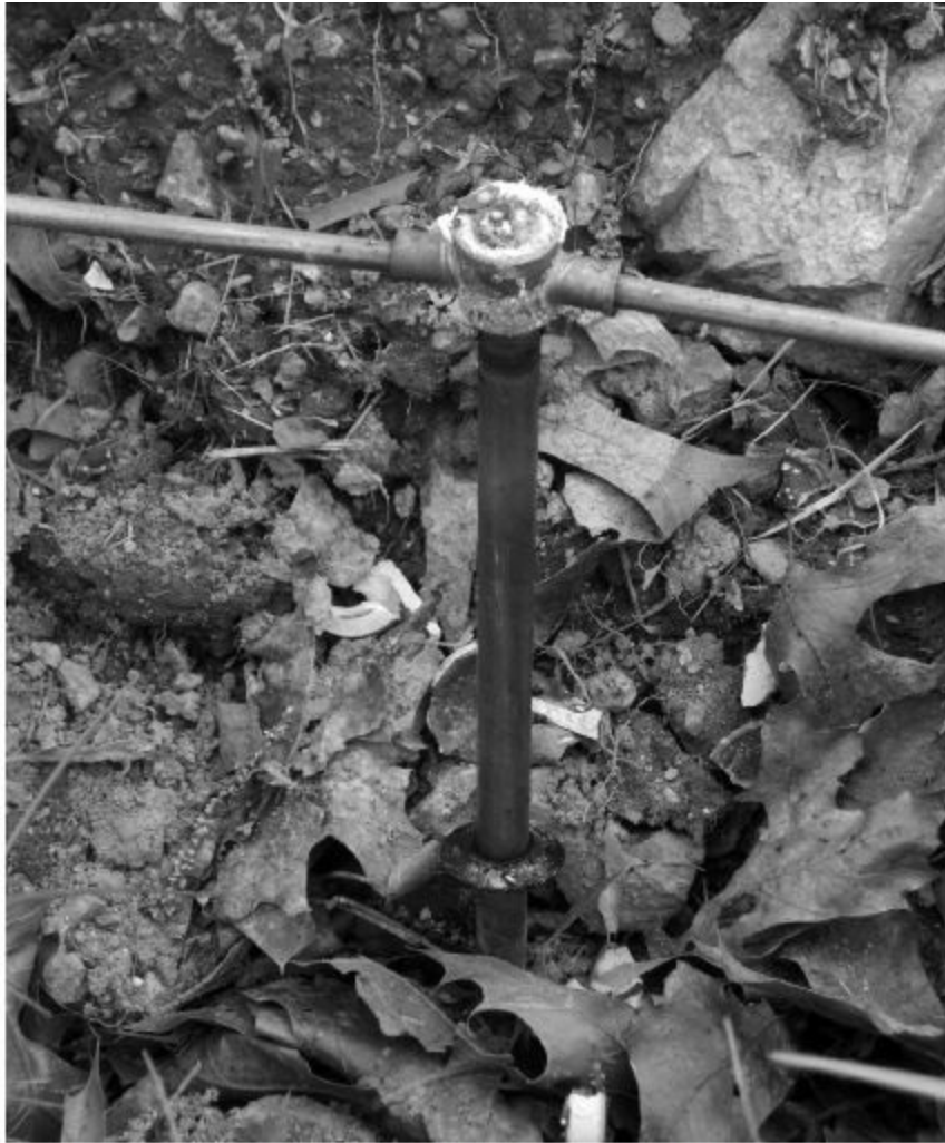
Figure 6.3 — A welded ground rod connection between #2 AWG copper wire and a 1/2-inch ground rod. This connection was then buried as part of a tower grounding system.
