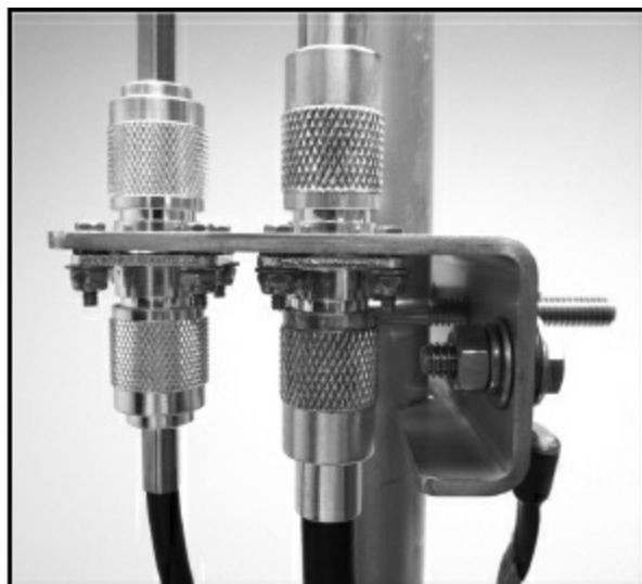
Figure 4.16 — A commercial coaxial cable grounding kit from DX Engineering (A). The same kit used to bond a pair of coaxial cables to a tower leg (B).
